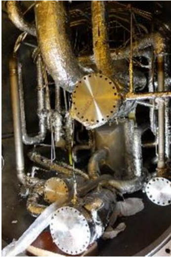
Warm-end of cold box modifications
