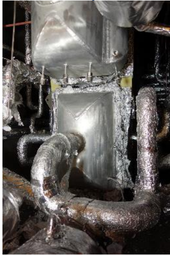
Heat exchanger tapings (taken out)
