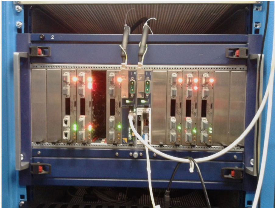
Fig. 5.1 The provisional crate installed with 6 production MP7s. The final crate, due Nov 19th, will have redundant power modules mounted in the rear (currently top centre). The optics are not yet cabled up.
