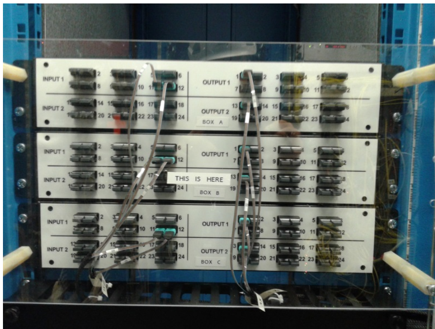
Fig. 5.2 The full mesh patch panel. It allows significant interconnect possibilities. The boxes shown here shuffle 288 fibres, but the technology used to construct them allows more than an order of magnitude more to be squeezed into the same space.
