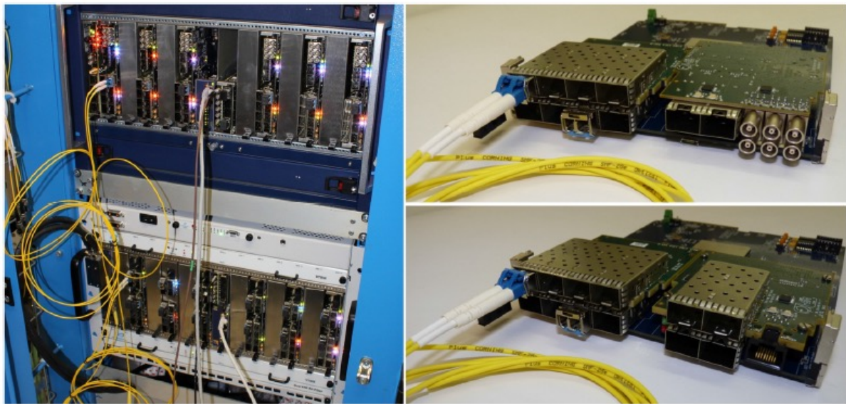
Fig 4.3 Left: TCDS demonstrator system installed in the CMS Underground Service Cavern at Point 5. Right: The two types of TCDS board, utilising the FC7 as carrier and different custom made FMCs to satisfy their respective specialised functions.
